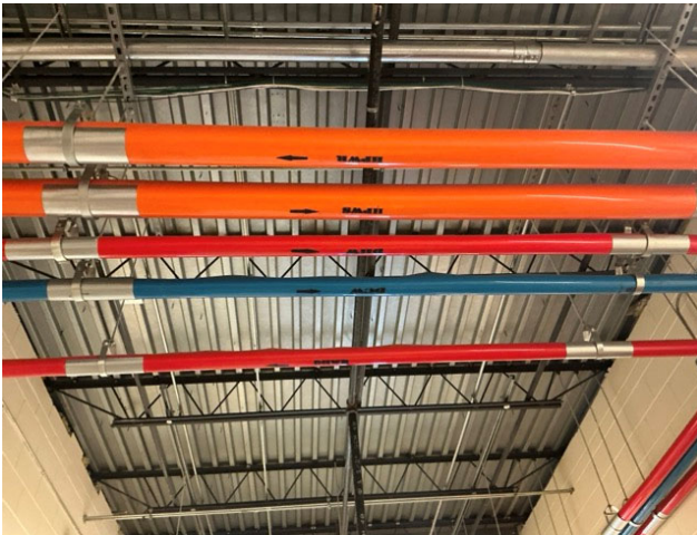
15 - DOMESTIC WATER PIPING
