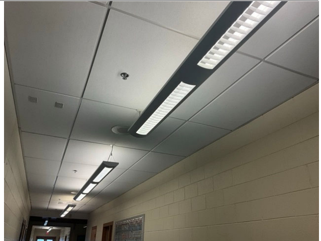
26 - INTERIOR LIGHTING SYSTEM
