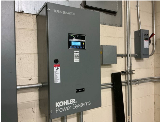
25 - AUTOMATIC TRANSFER SWITCH
