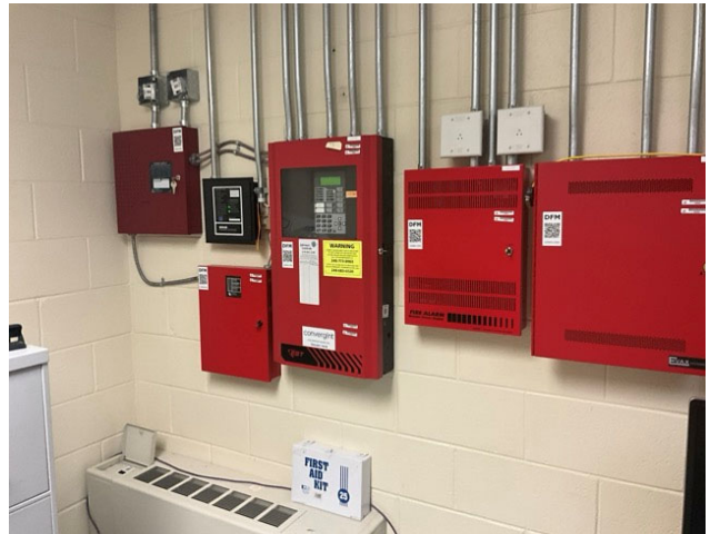
28 - FIRE ALARM PANEL
