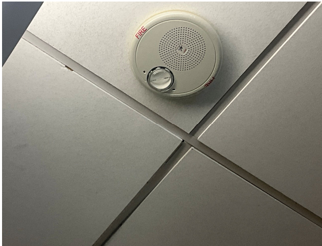
27 - FIRE ALARM SYSTEM
